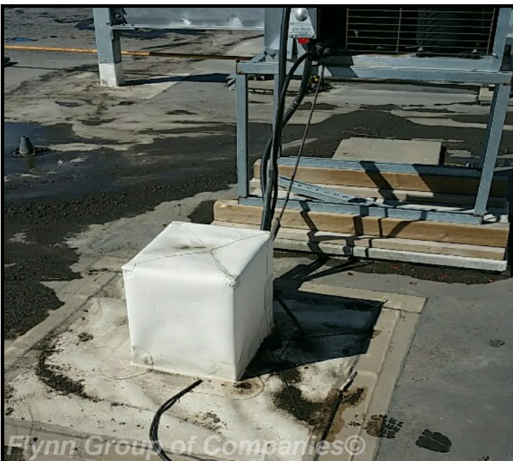
Section_A: Curb requires cap flashing, 14.5 by 16.5
