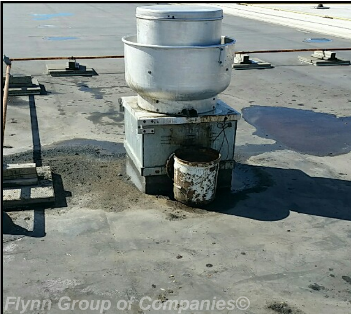
Section_A: Grease vent needs new trap and cleaned around vent.
