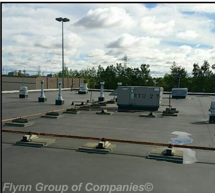
Section_A: View of RTU 27
