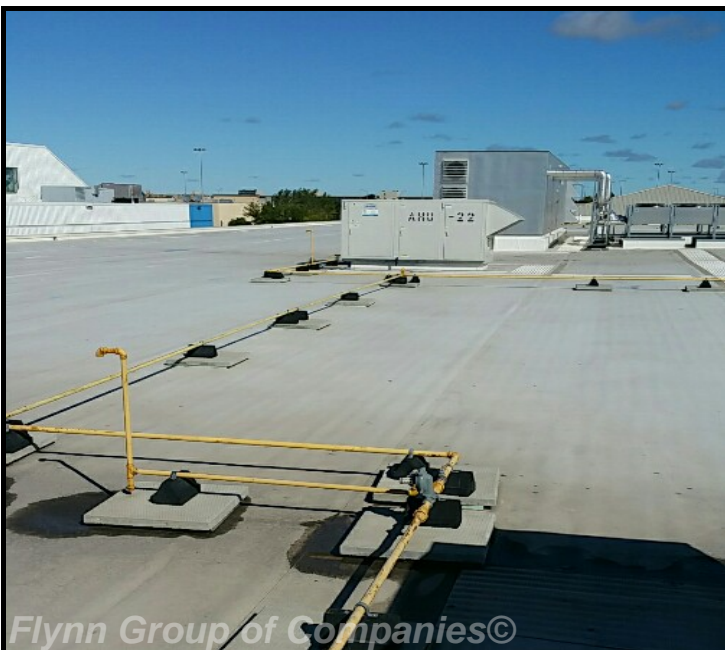
Section_B: View of gas lines running into AHU 22
