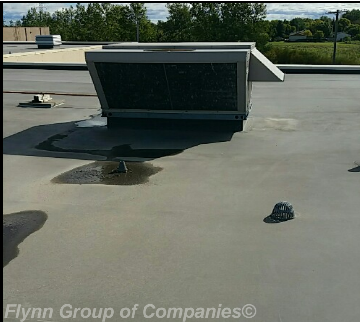
Section_A: Will clean and put screen back on.
